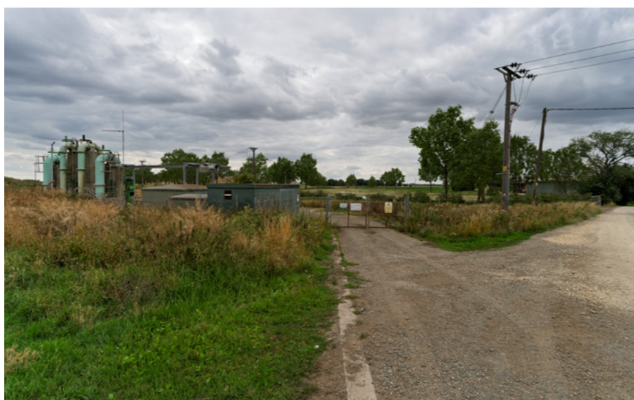
For illustrative purposes only. View from Levitt's Drove of the proposed location for the river abstraction and treatment facility and pumping station.
