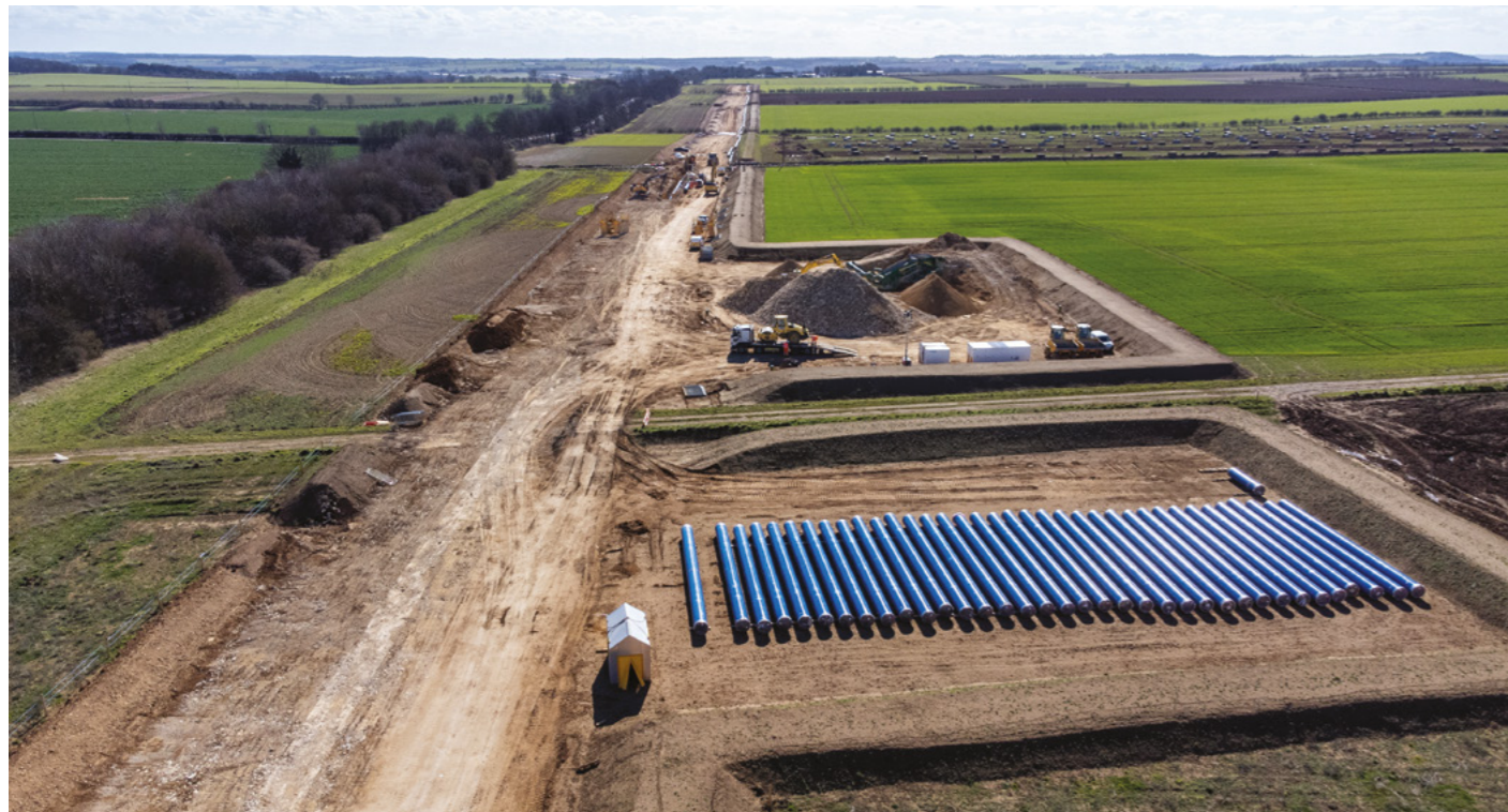
Example of a lay down area from our Strategic Pipeline Alliance project.
